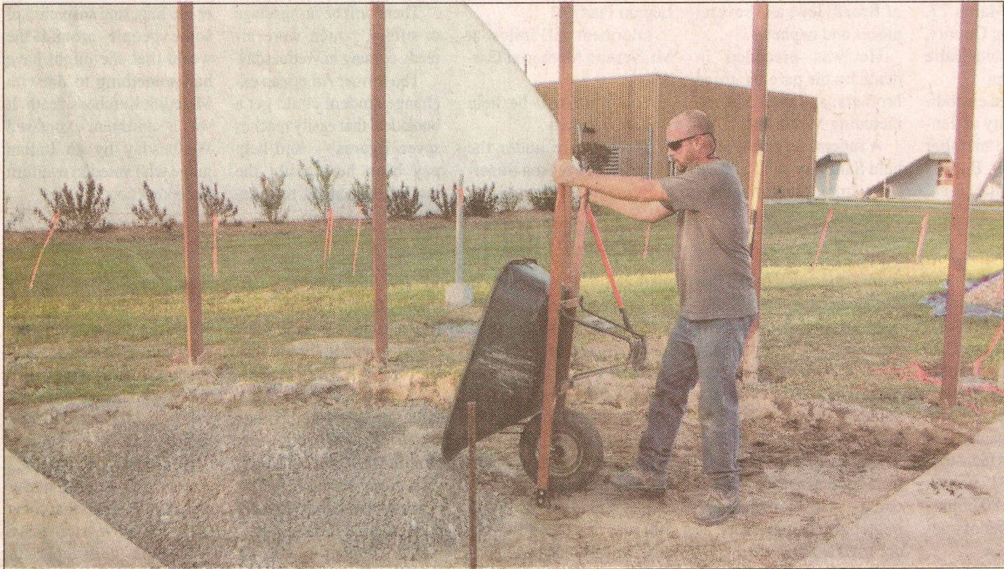
Tony Donoho of Lipps Construction lays gravel for the Jefferson County Heroes Memorial being constructed at the Mt. Vernon Outland Airport. The memorial will be completed and dedicated on Oct. 15 at the EAA Little Egypt Fly-In.
